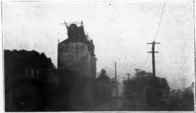
Freight Cars Loading at Concrete Storage Bins. Drag Washer May Be Seen on Top of Bins at Right of Screen
